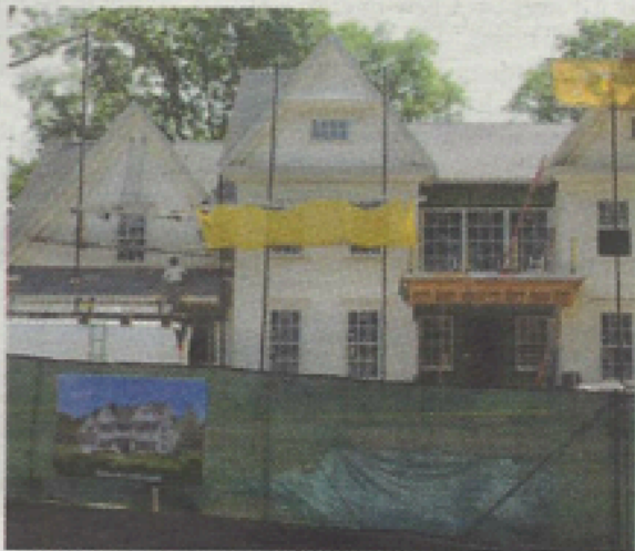
Photo 3: The new "healthy home" currently under construction at 8 Kent Road in Scarsdale. Photo Credit: Christopher Banuchi.
